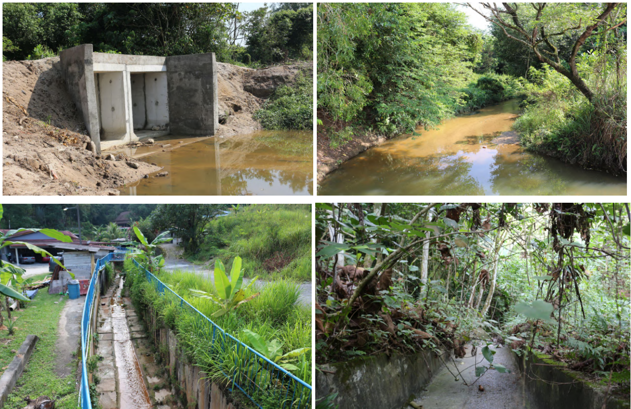
Figure 24. Existing culverts and drainage networks serve as ecological linkages for wildlife.
